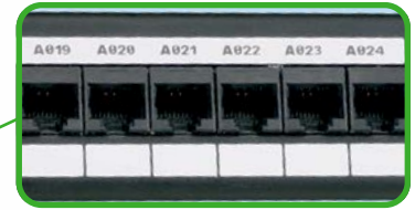
Patch Panel / Face Plate Labels
